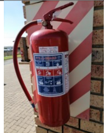
Photo 3: Un-serviced Fire Extinguisher
