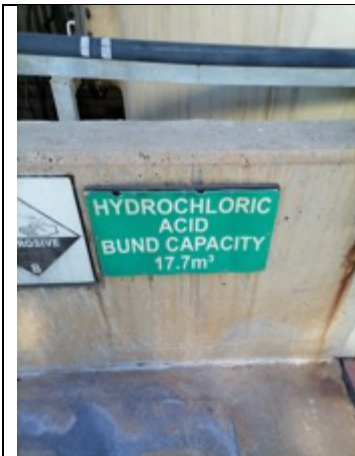
Photo 10: Example of chemical storage bunded area.
