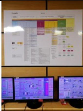
Photo 2: Example of SCADA system
