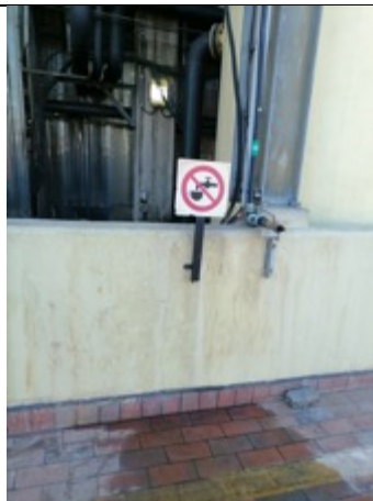
Photo 11: Example of warning signage (Do not drink).
