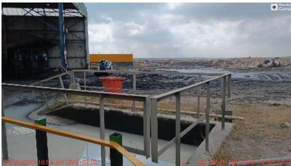
Photo 17: HDV Washday, blockage of sumps
