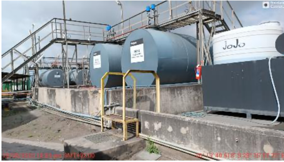
Photo 19: Hydrocarbon Storage on bunded surfaces
