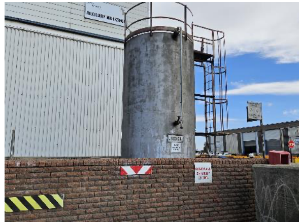
Photo 4: Bunded oil storage area at Auxiliary workshop
