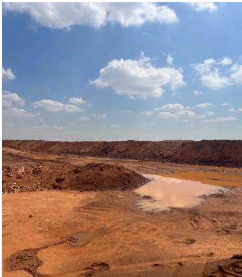
Figure 13: Water pooling on internal access road
